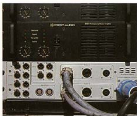
Crest 8001 amps above SSE input/output panels.
